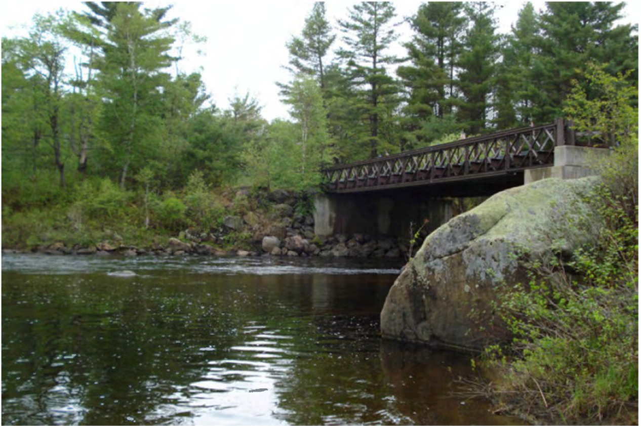
Photo 1: Polaris (Iron) Bridge over the Hudson River. Taken from the east shore, looking west.
