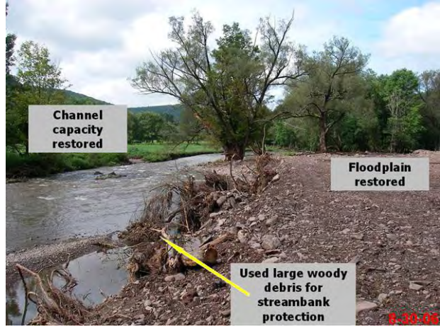
Figure 3.18 Stream construction using Regional Bank full Hydraulic Geometry values, typical cross-section and root wad.
